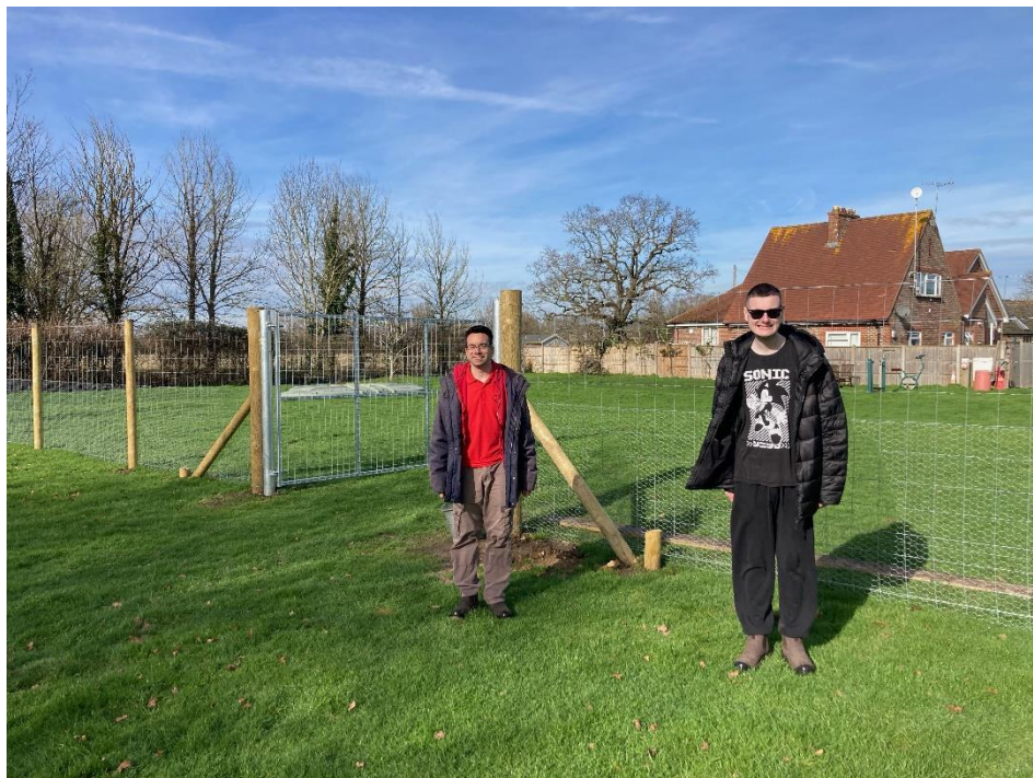
Most of the fencing is up. It should open later in the year.
